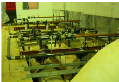
Figure 12 - Chilled water piping
